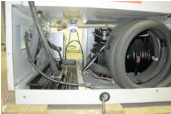
Rear Access Panel Removed
