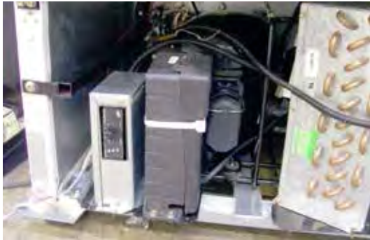
Safe-NET III Controller Location
