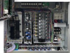
Shown: Main Electrical Panel
