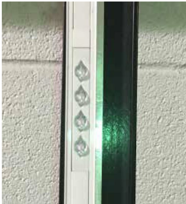
Figure 5. Interior View of End Fixture
